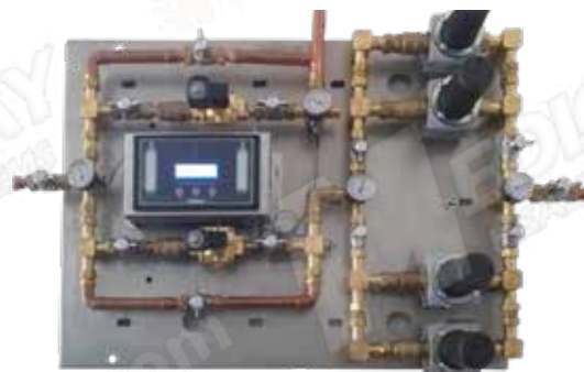
LIQUID OXYGEN TANK & AUTOMATIC MANIFOLD SYSTEM CONNECTION PANEL
