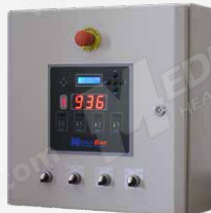
AGS PLANT CONTROL PANEL
