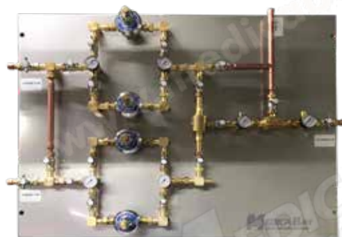
TWO LIQUID OXYGEN TANKS & AUTOMATIC MANIFOLD SYSTEM CONNECTION PANEL
