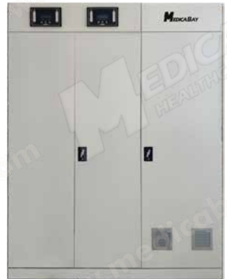
TRIPLEX EMERGENCY CABINET
