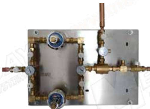
LIQUID OXYGEN TANK & AUTOMATIC MANIFOLD SYSTEM CONNECTION PANEL
